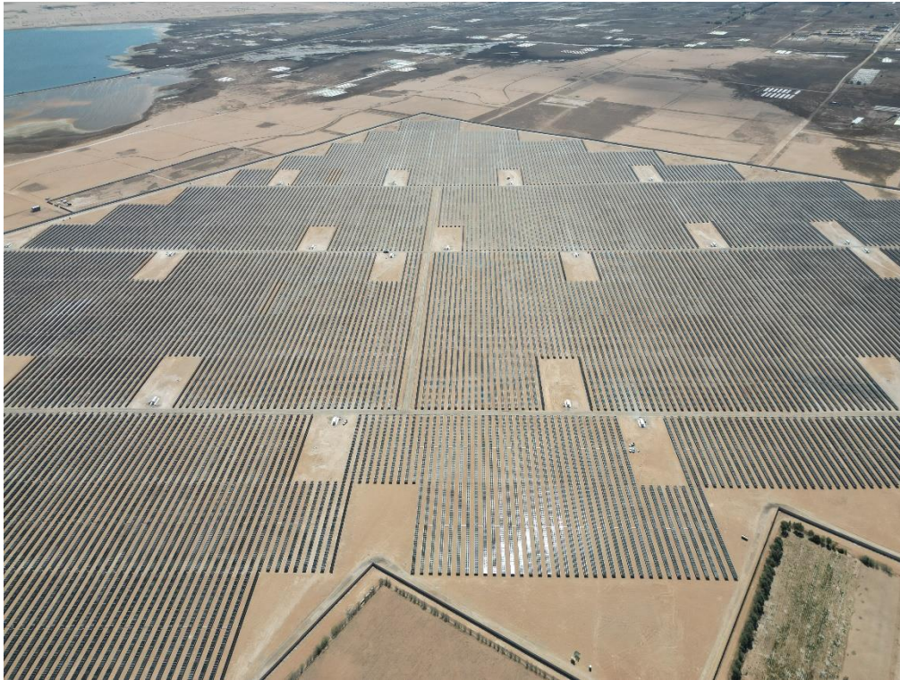
Yinson Renewables' Matarani Solar Plant located at Arequipa, has one of the highest photovoltaic (PV) power potential in Peru.
